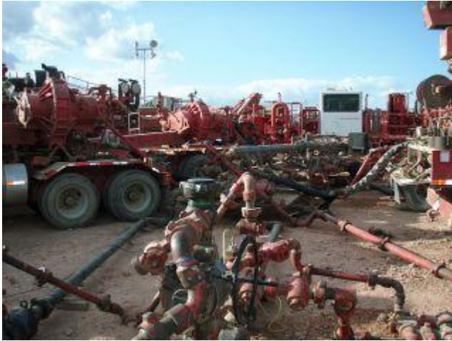
"Halliburton Fracturing Operation in the Bakken Formation, North Dakota". Bild: Joshua Doubek/CC BY-SA 3.0
